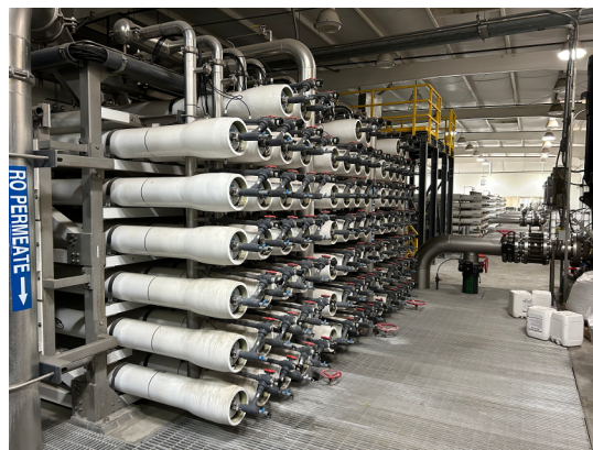
Figure 1: A photo of an RO train at Chino Desalter Authority
